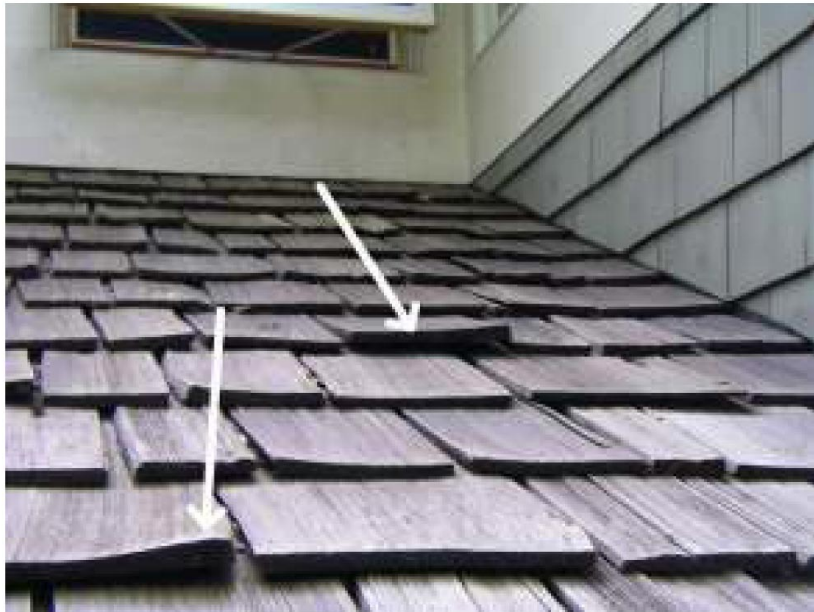
Arrows show normal cupping of cedar Shake shingles. However, more advanced cupping is a problem and the shingles should be replaced by the contracted roofing company that specializes in treatment and repair of these wood shingles.
