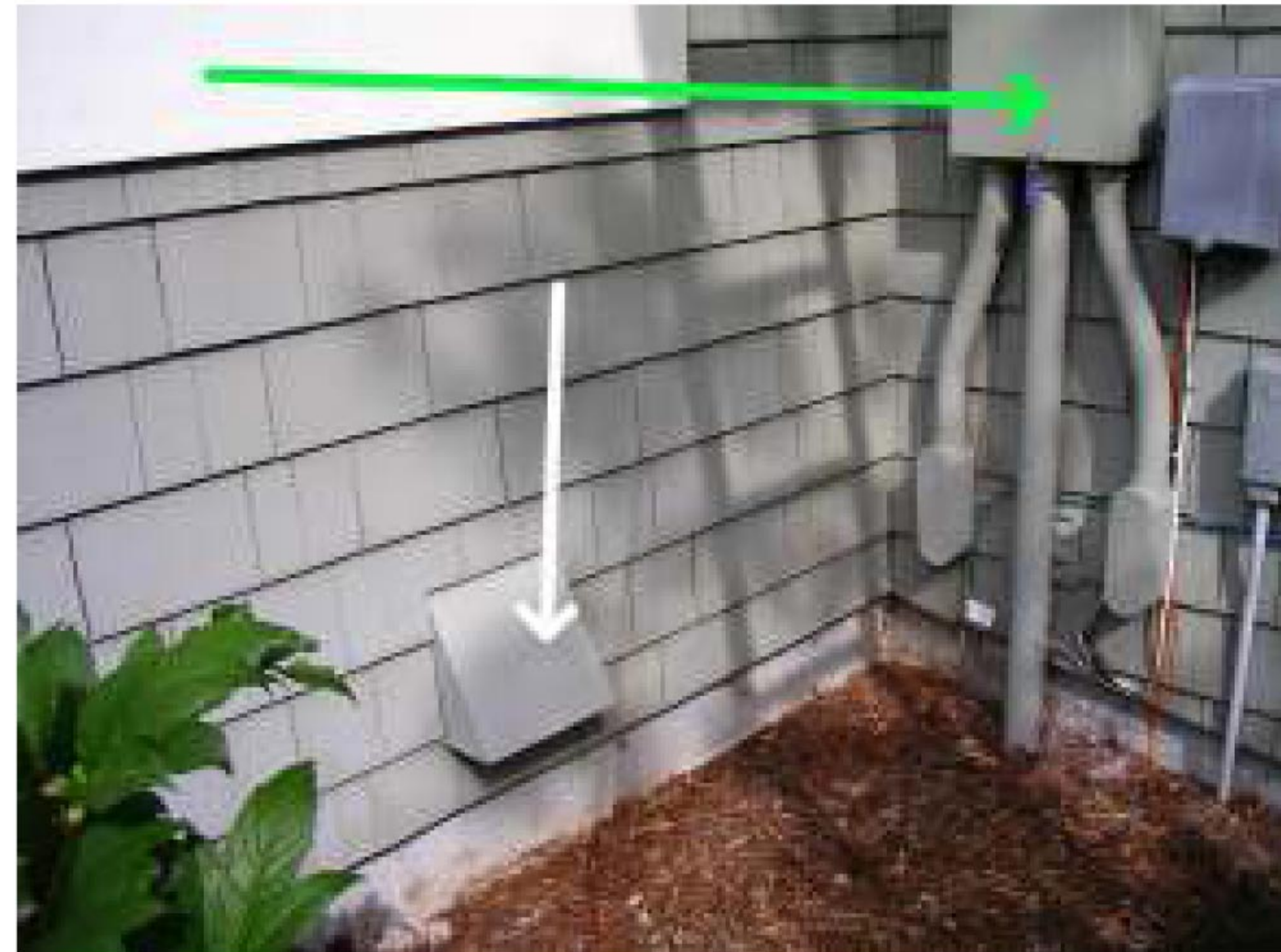
White arrow shows one of the fresh air vents for the furnace and water heater that must be kept clear of obstructions. Green arrow show electrical service entrance.
