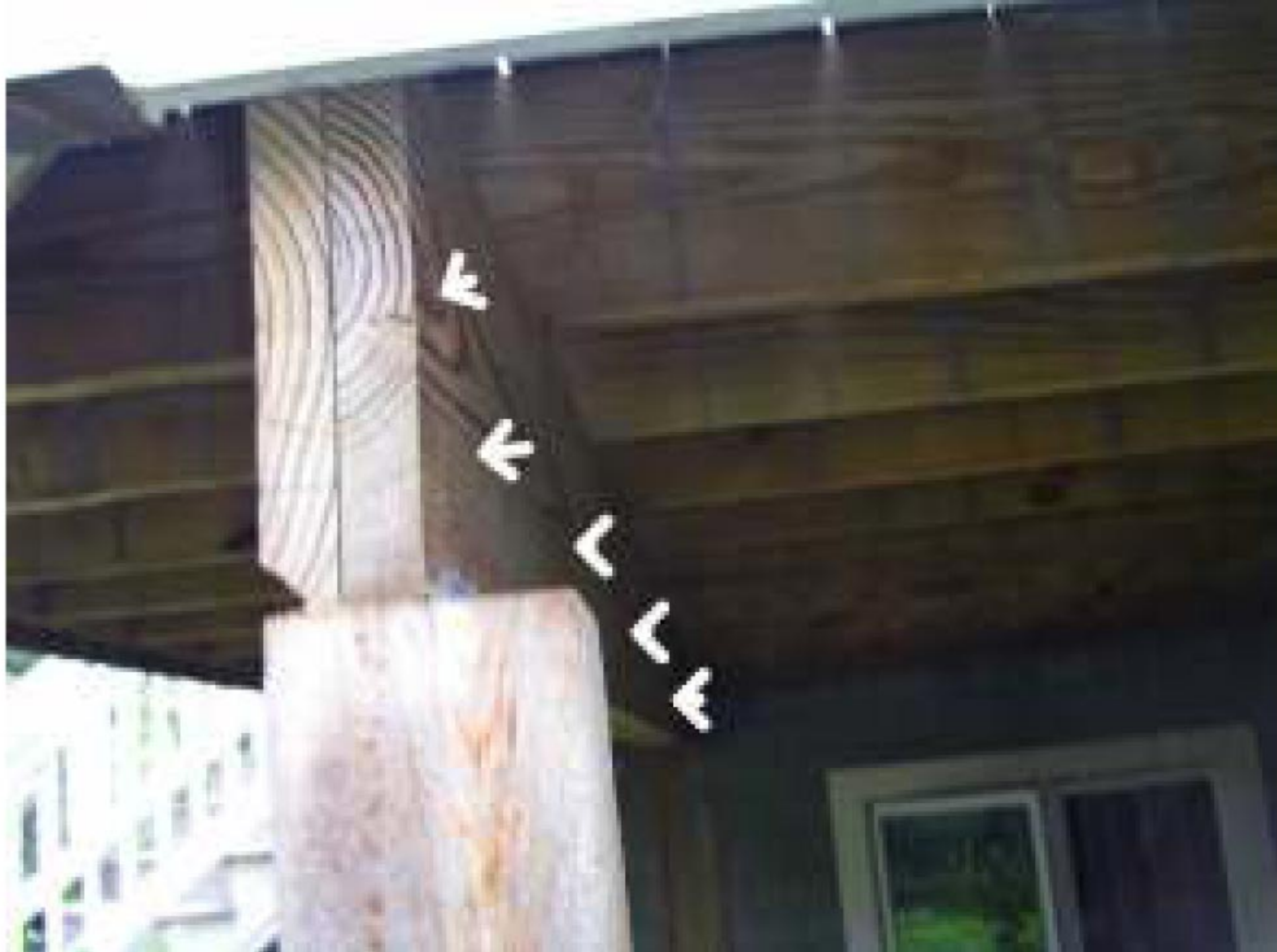
This deck beam will benefit in years to come from proper carriage bolts that will counter act the wood's tendency to warp, move, and deteriorate from water at the facing adjacencies.
