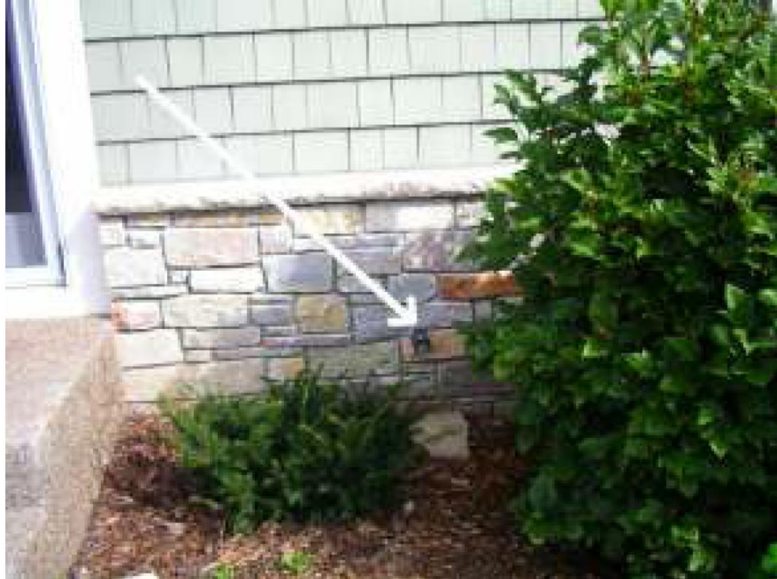
This west side hose faucet IS freeze-protected.
