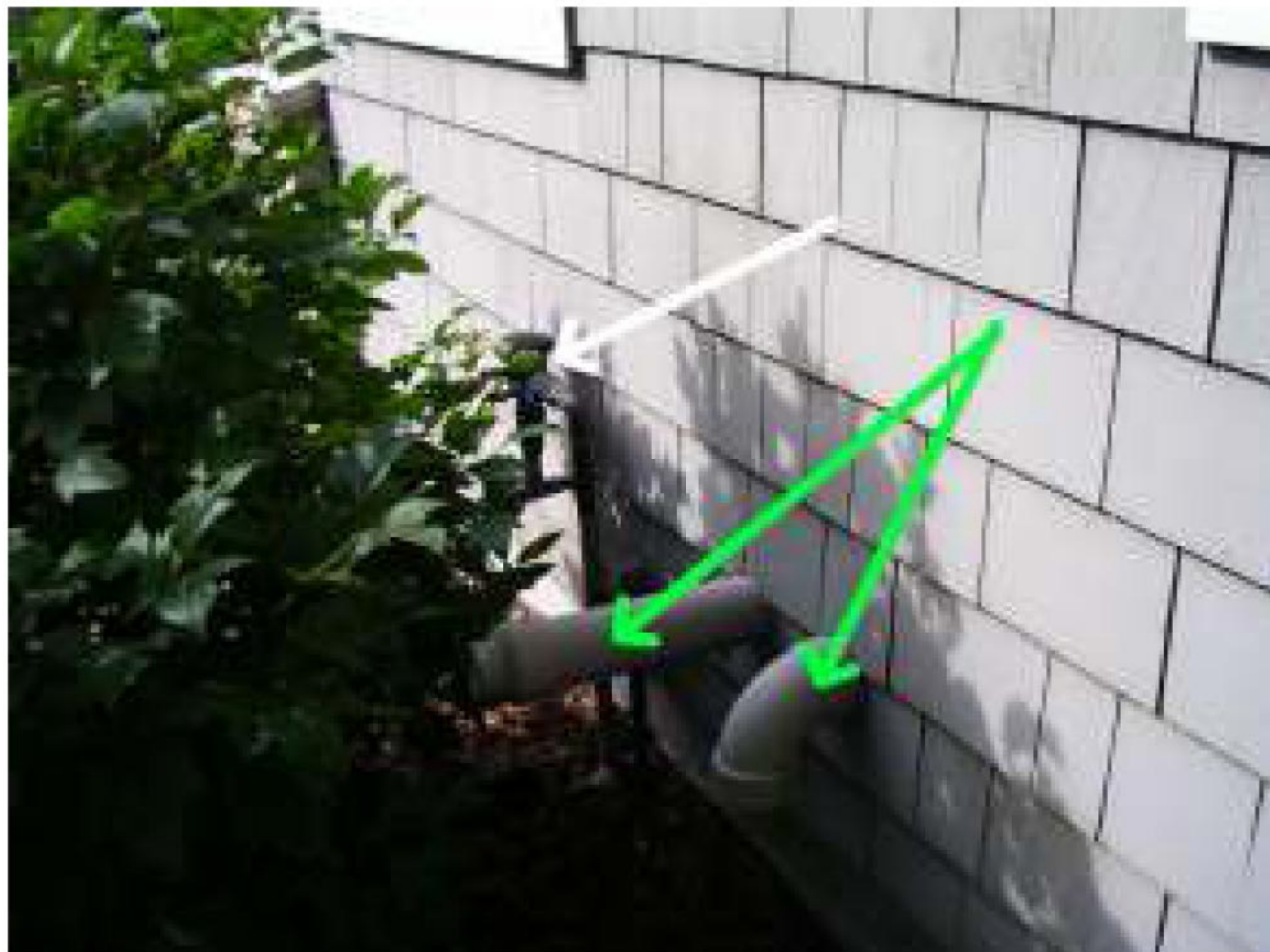
White arrow shows proper design and placment of the sprinkler system backflow preventer valve. Green arrows show furnace exhaust and fresh air
