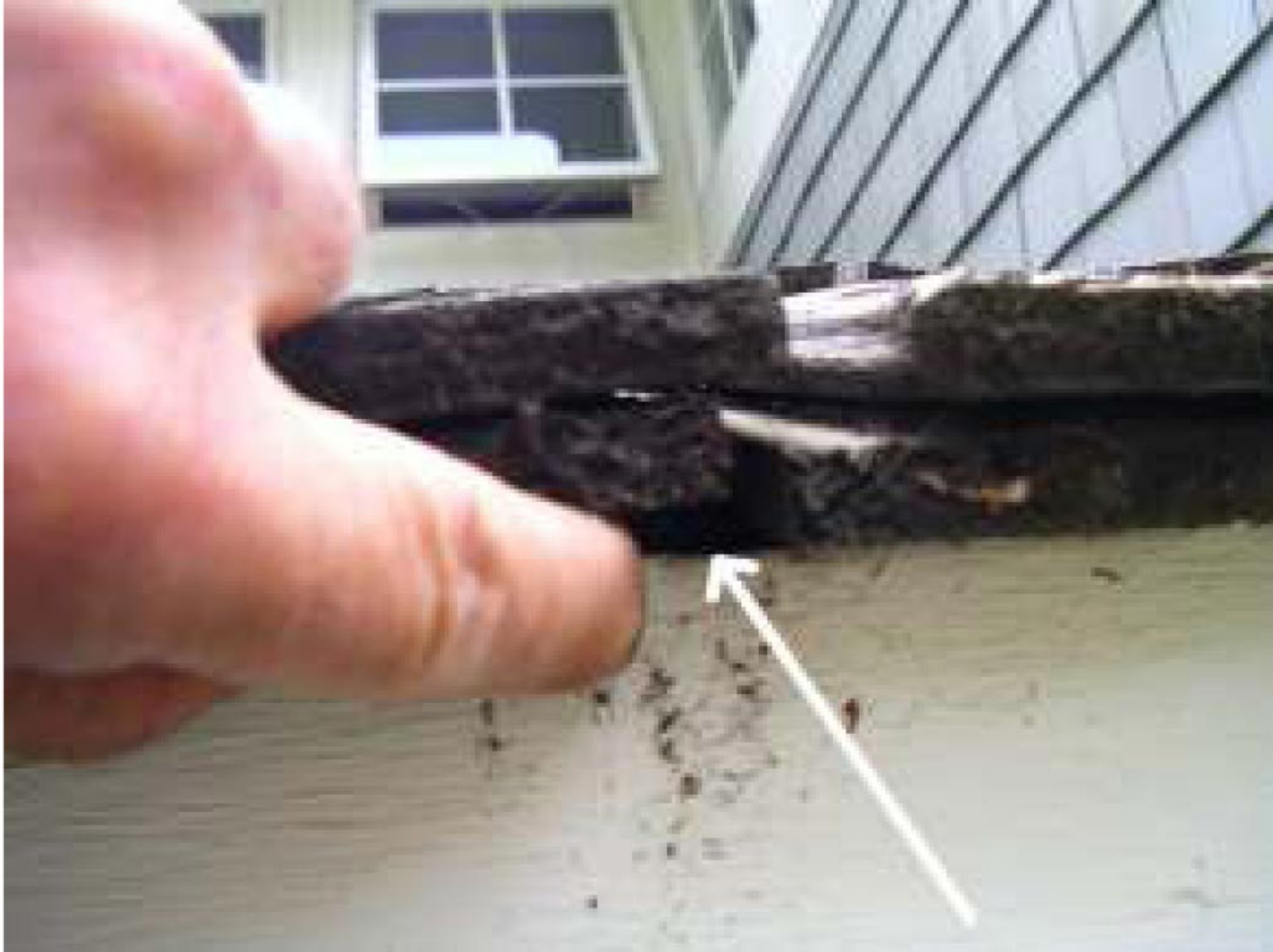
No drip edge here. Not absolutely required, but would have been an effective prevention against water intrusion at the interior of the roof assembly. Monitor. This drip edge can be added.
