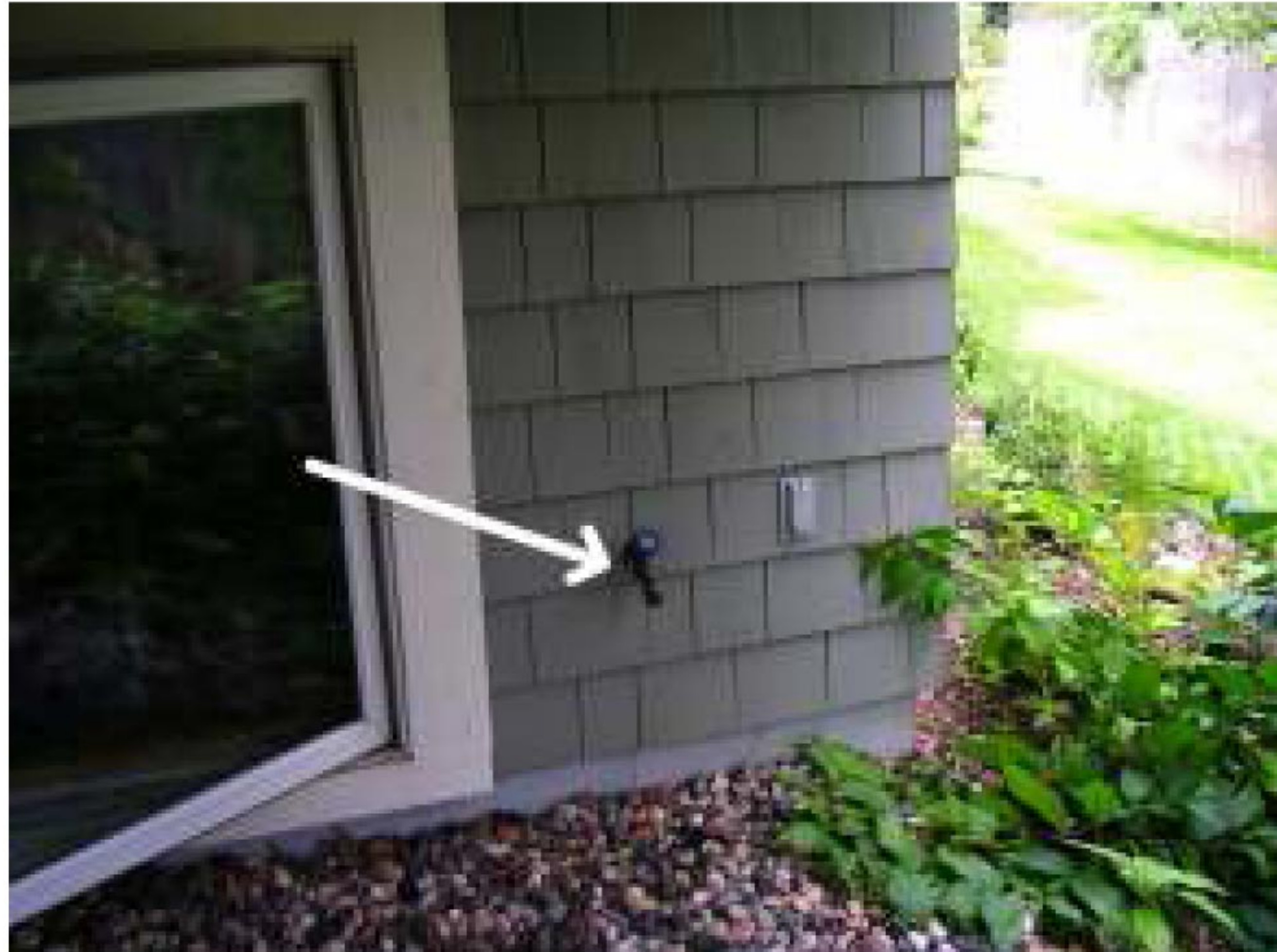
This south side hose faucet under the deck appears NOT freeze protected; it will have to be turned off and drained each fall.
