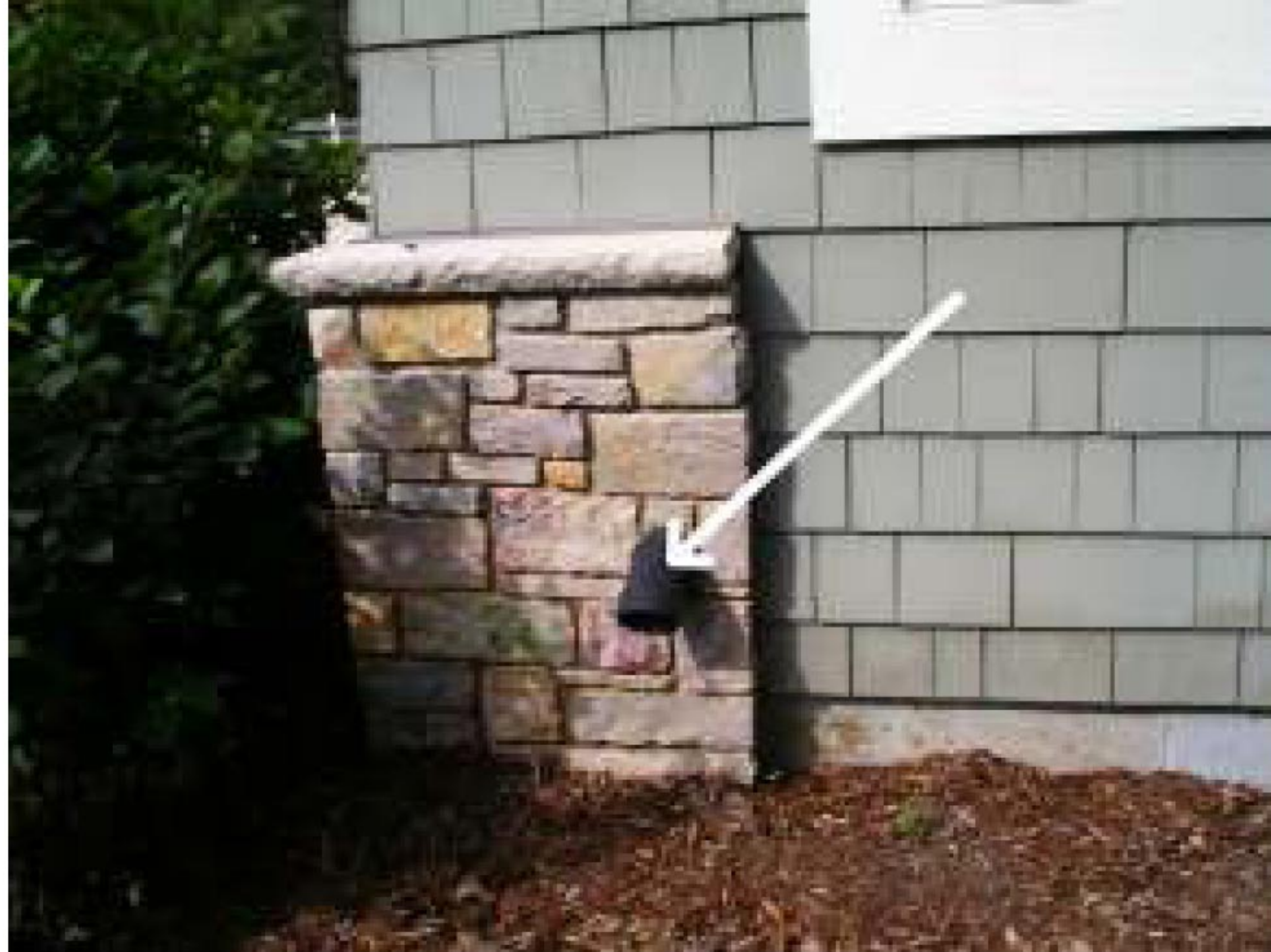
Arrow shows water heater exhaust that must be free of obstruction.
