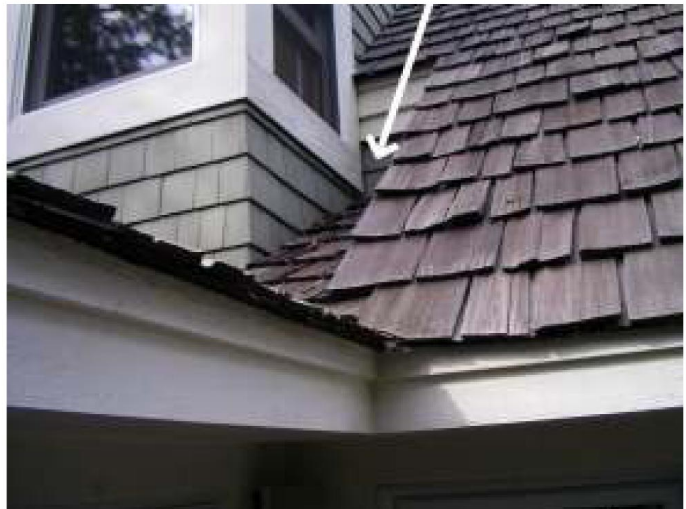
Arrow: just one of the areas where snow and ice will gather. Monitor for build up; watch for interior staining; take action as needed to prevent damage to interior. Proper heavy duty flashing and mambrane not visible here.
