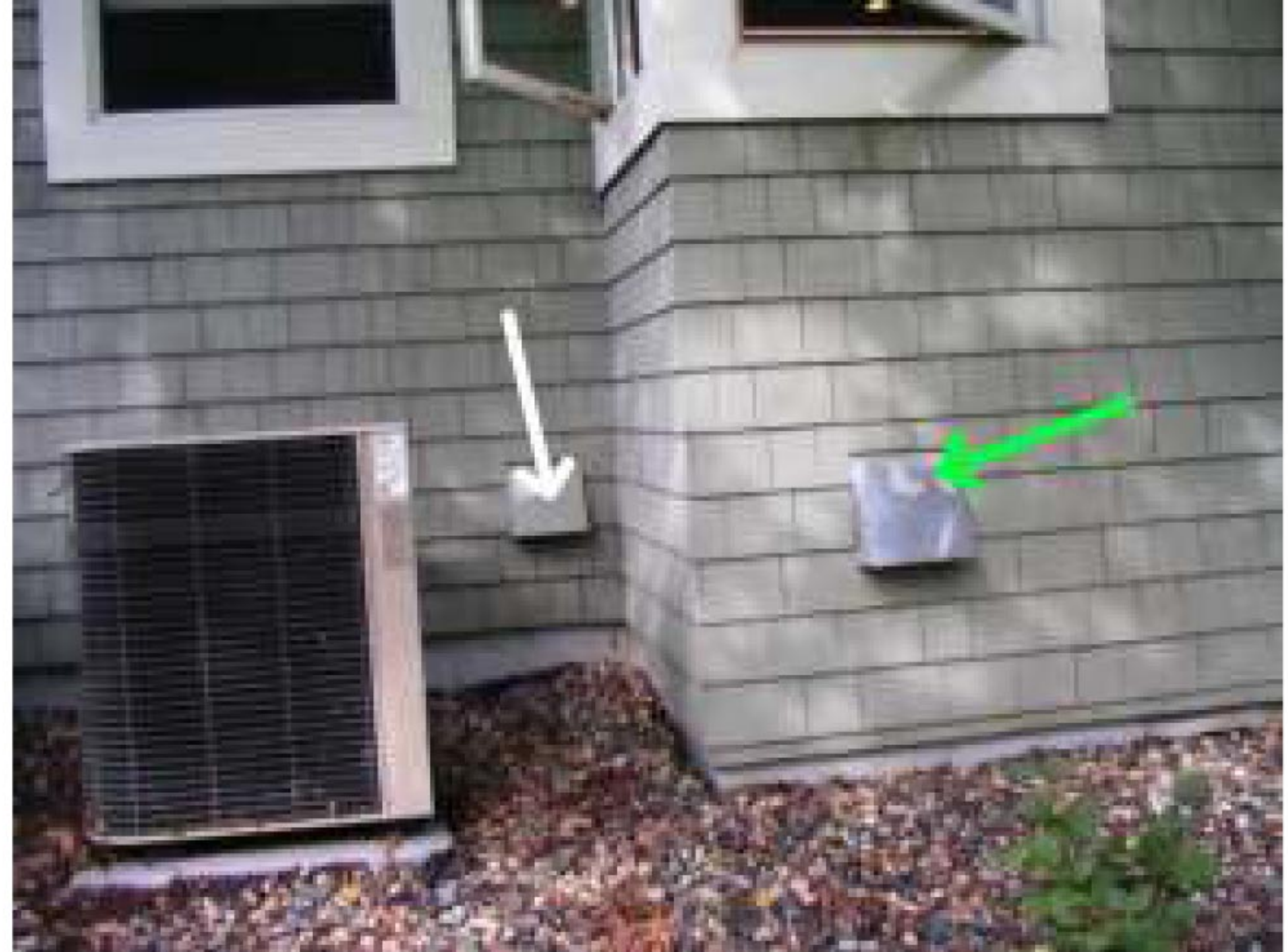
White arrow: vent for the air-to-air heat exchanger. Green arrow: fresh make up air for the furnace and water heater. Keep both obstruction free.
