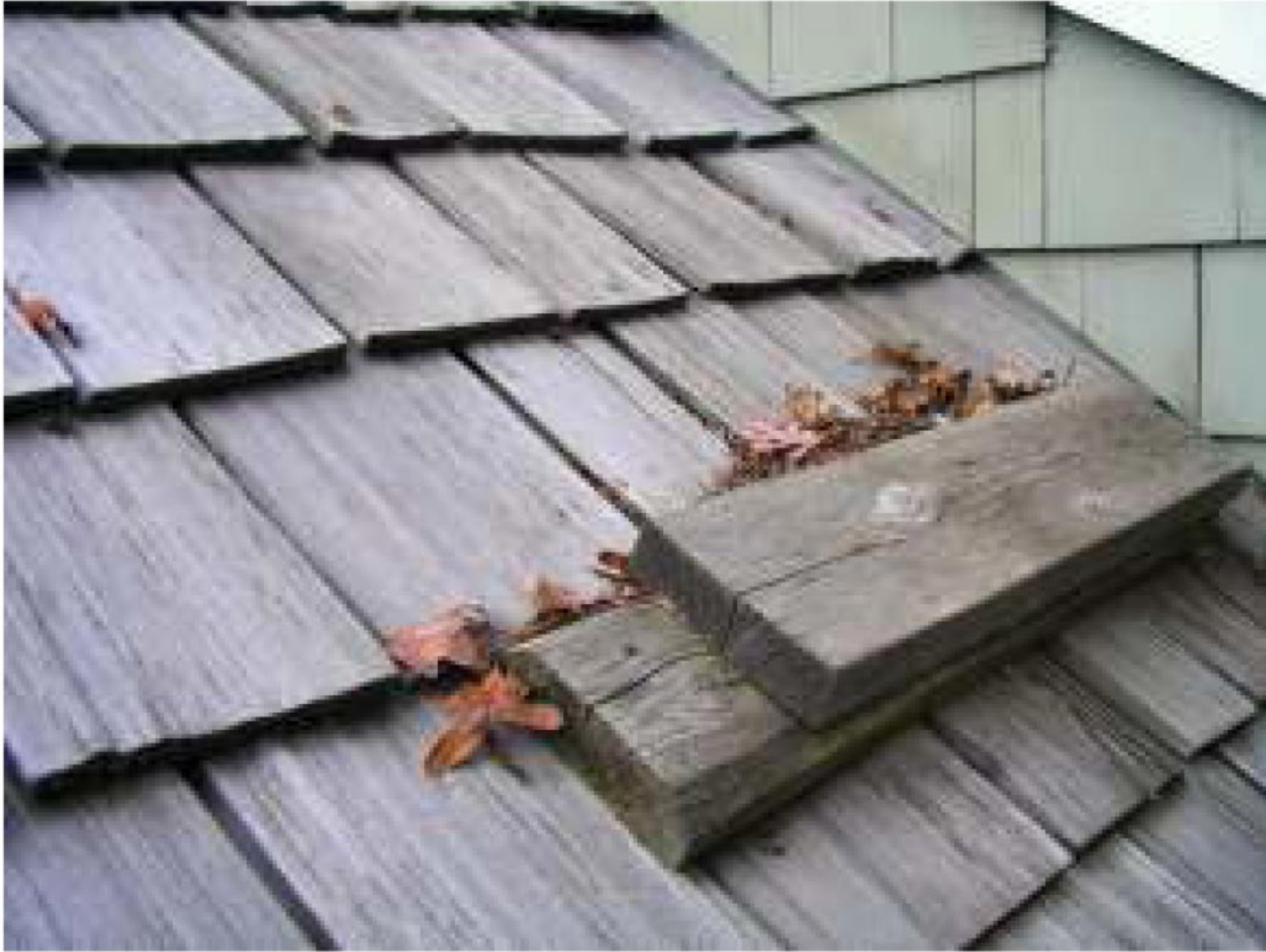
Roofers left this climbing ledger in place. Recommend removal.
